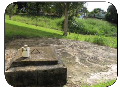
Keep septic tanks sealed.
