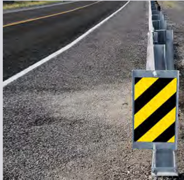
Delineate Roadside Hazards
