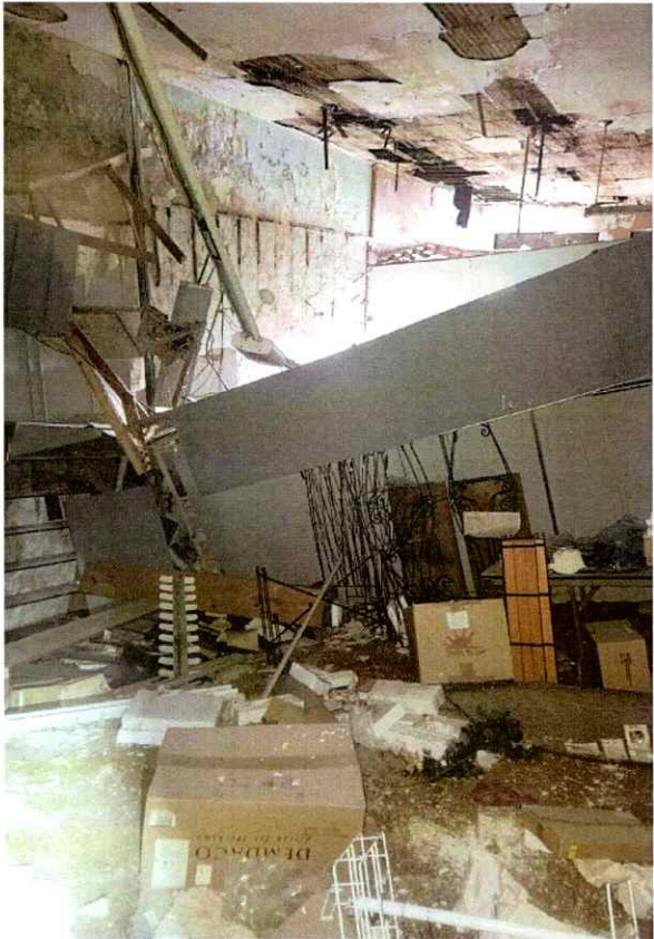
Area 3 Floor Collapse viewed from 3rd Floor
