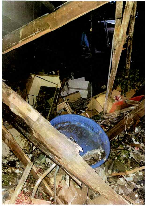
Area 5 Floor Collapse viewed from 2nd Floor
