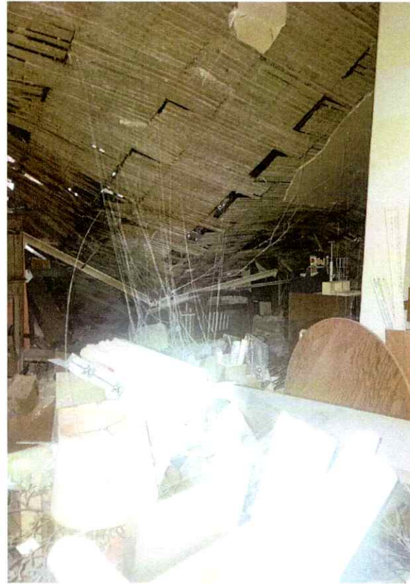
Area 3 Floor Collapse viewed from 3rd Floor
