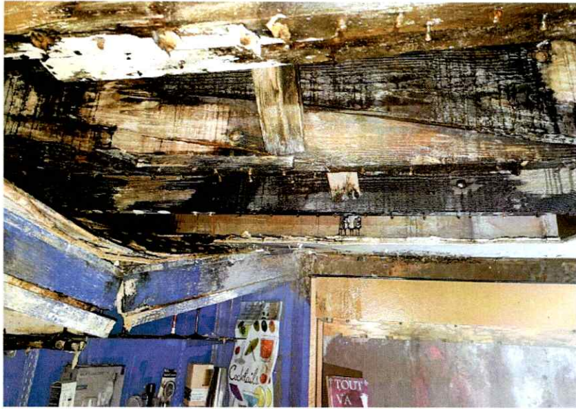
Area 1 Floor Joist Failure viewed from Mezzanine
