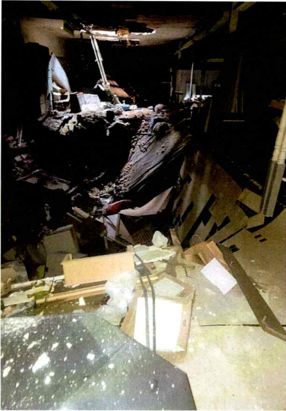
Area 5 Floor Collapse viewed from 3rd Floor
